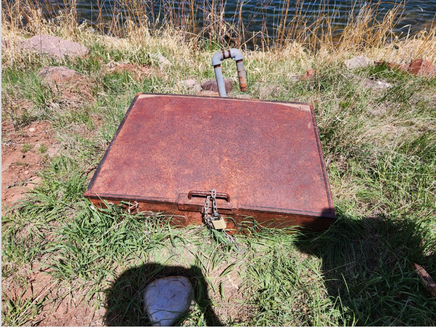
Outlet Operator Vault
