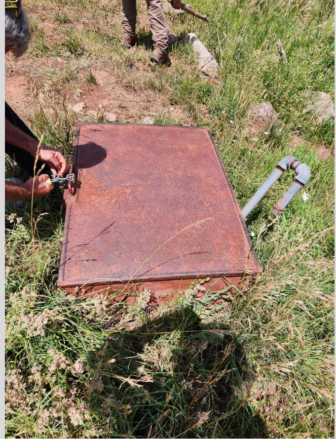
Outlet Operator Vault
