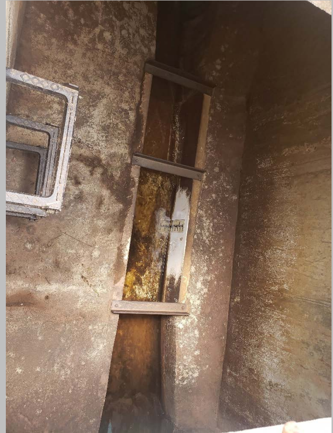
Parshall Flume in Vault
