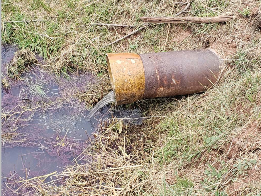
CIPP Lined WSP Outlet Conduit – Note Increased Gate Leakage
